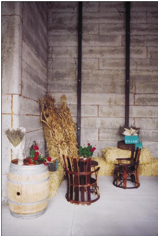
Exposed walls in the covered event area show the Perform Wall building panel blocks made of recycled polystyrene and cement, providing up to R-26 insulation value.
